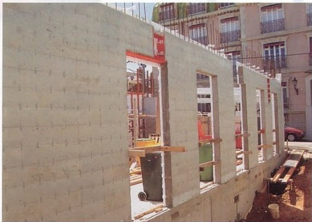
The exterior face of the wall after the plastic planks have been stripped away.
