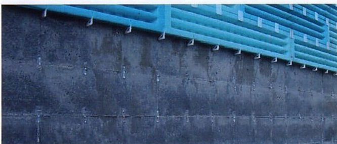
In-situ concrete wall after the ICF plastic formwork has been stripped out.
